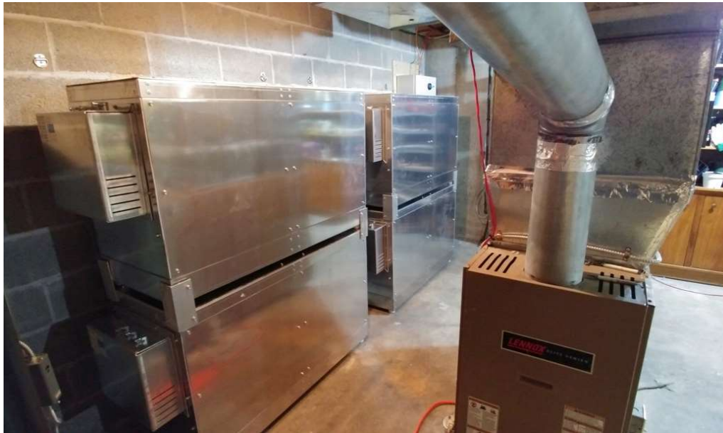
Neothermal ETS 2019 Prototype Integrated with Oil Forced-Air Furnace in Halifax, NS, CAN
